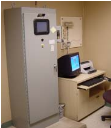
A typical SCADA master control system consists of PLC, radio, desktop PC and printer.
